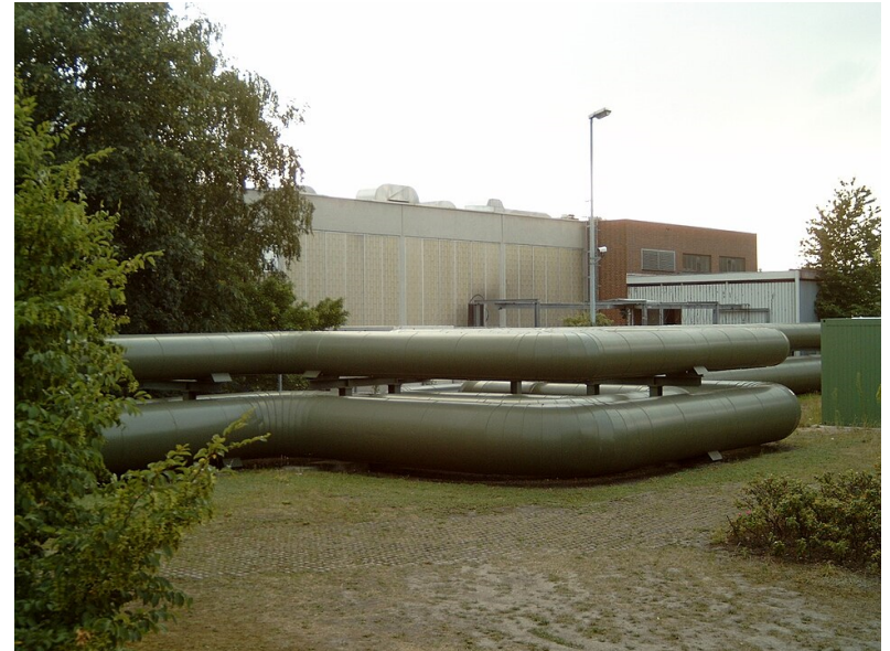
community power plant Hanover (Germany), district heating main pipes with U-bows for expansion compensation
